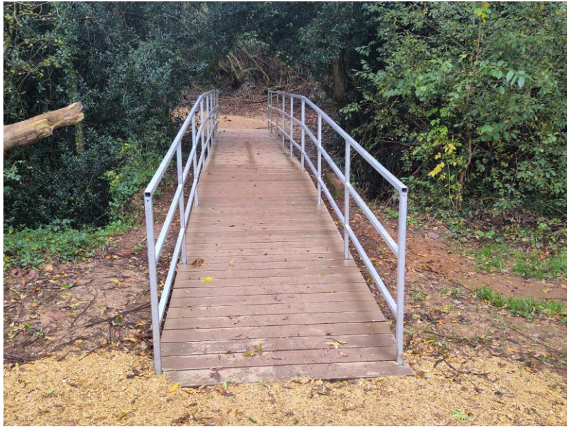
New foot bridge over existing culvert of unknown safety
