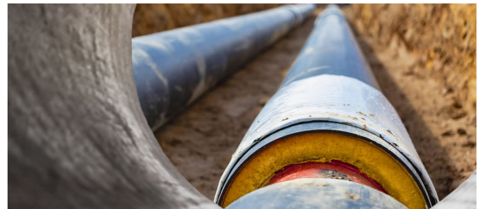
District heating has been delivered at Monkerton, Exeter.
