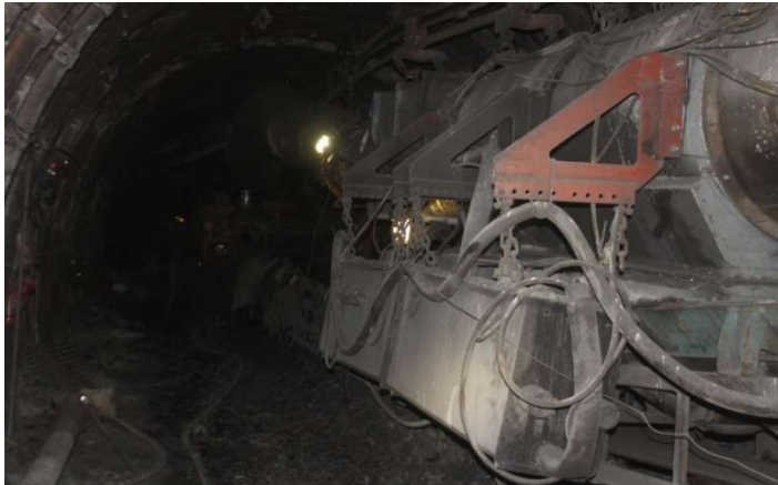
Figure 15 Dust collector OD-1000/1000 in the Knurów underground mine.
