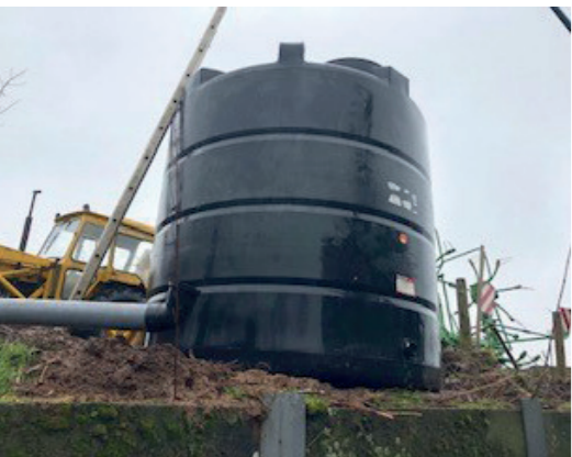
Figure 3 New water storage installed on a farm on the Dart to store dirty water and reduce the risk of nutrient loss to surface water; photo by DWT.
