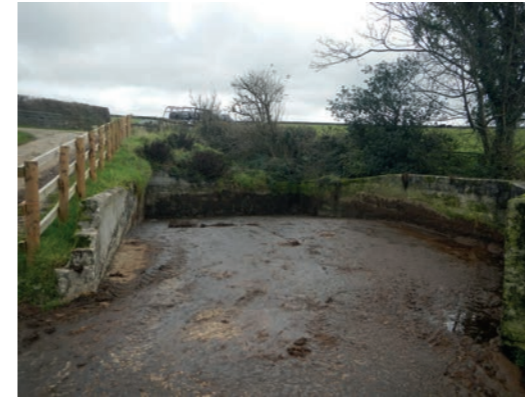
Figure 8 Before (left) and after (right) the installation of a new slurry storage with concrete base; photo by FWAG.
