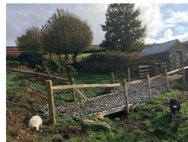
Figure 10 Re-siting of access to field and watercourse fencing installed to prevent livestock access; photo by Devon Wildlife Trust.
